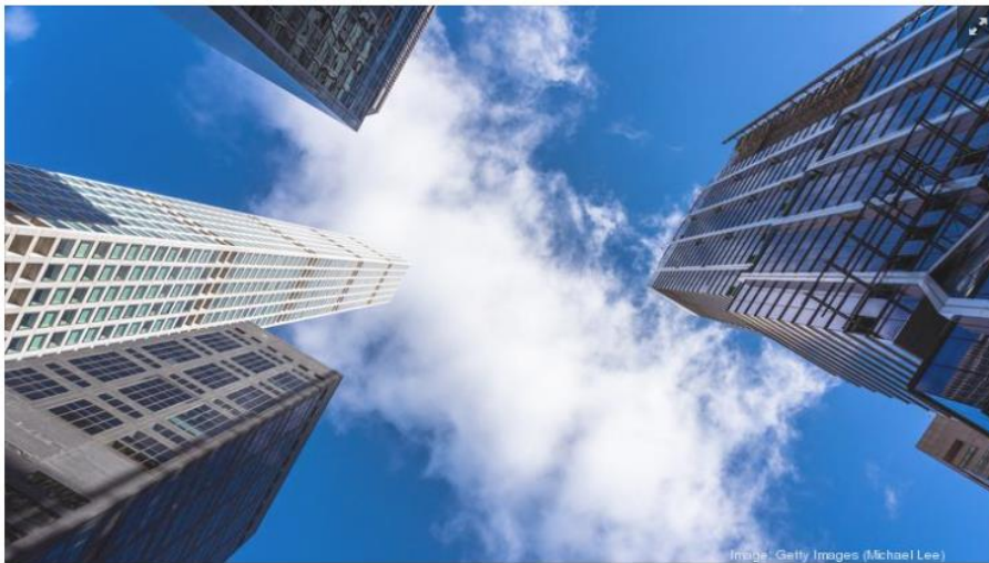
425 Park Ave. is under construction between East 55th and 56th streets. GETTY IMAGES (MICHAEL LEE)
