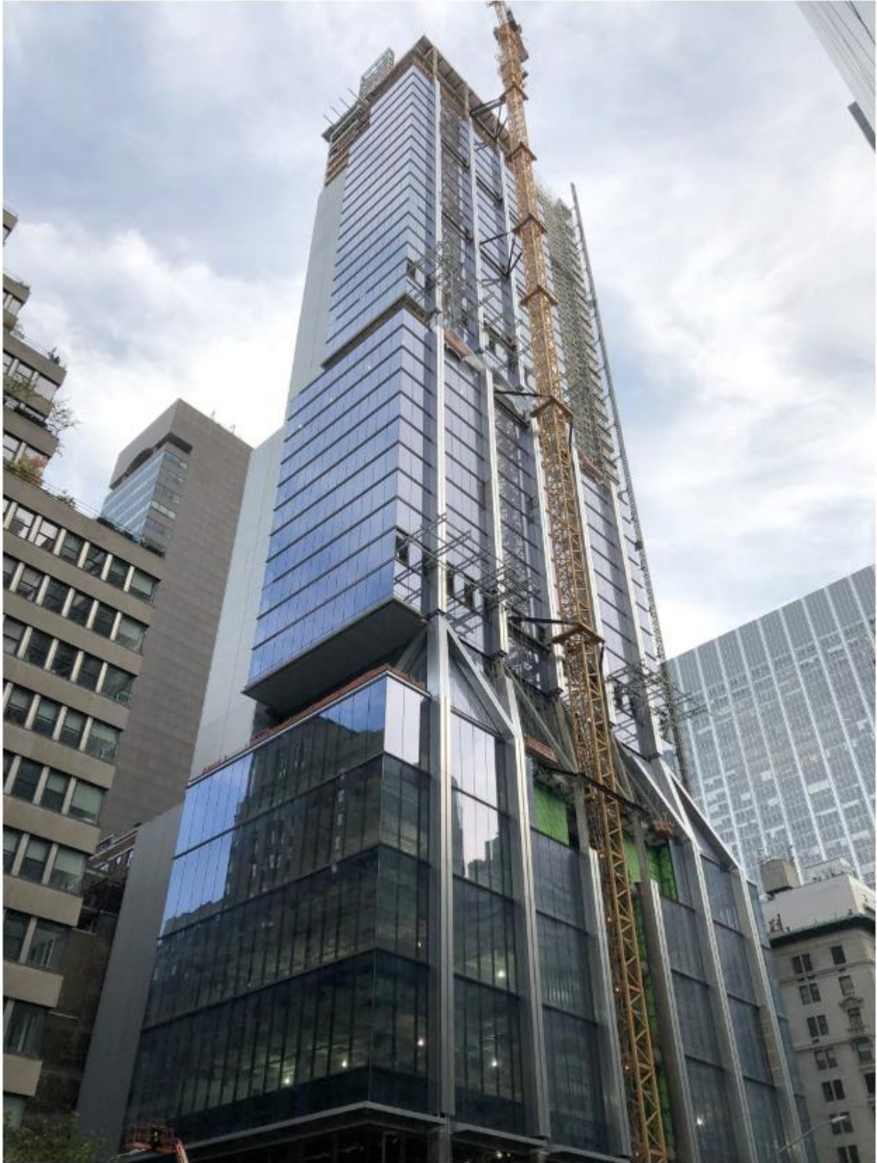
Looking up at the main Park Avenue elevation. Photo by Michael Young
